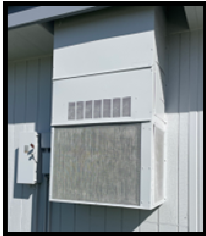
View of existing BARD unit at D-108
