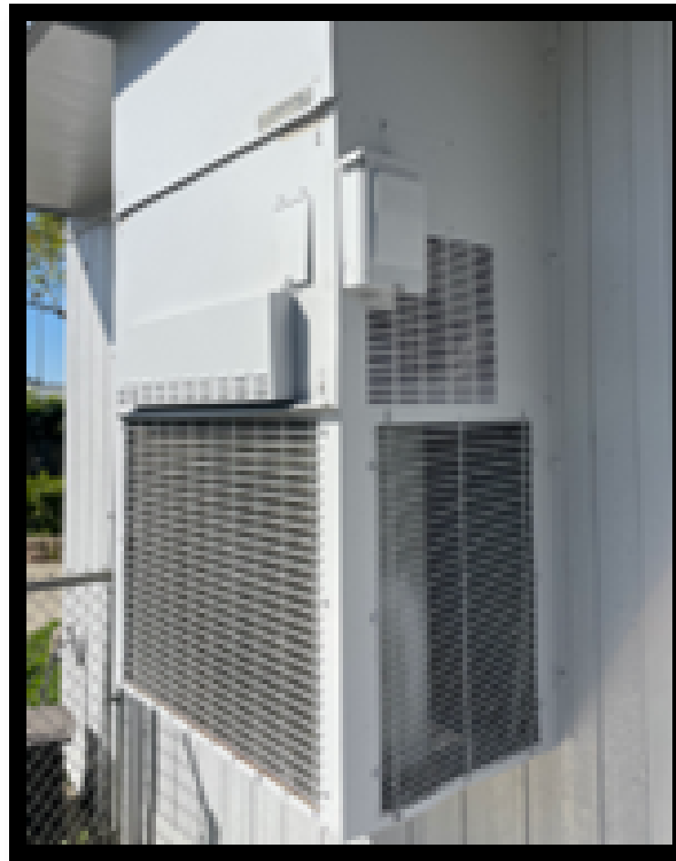
View of existing Crispaire unit at C-110
