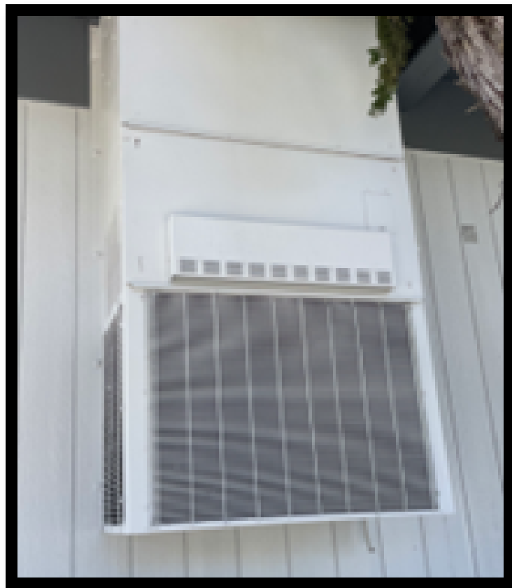
View of existing Marvair unit at C-111
